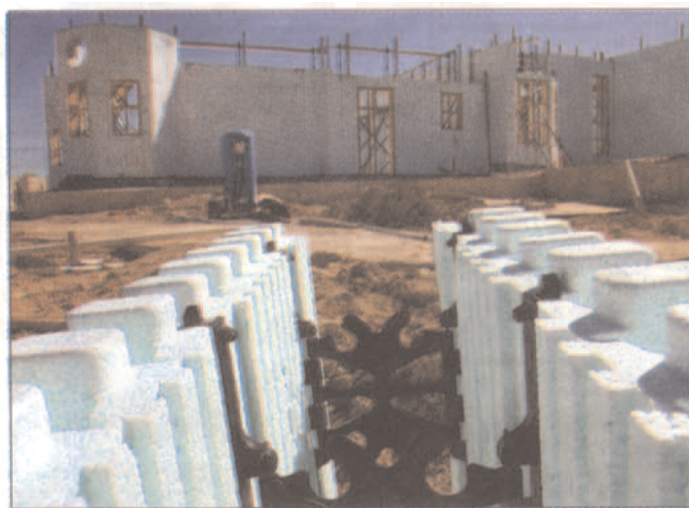
Concrete is poured between these plastic forms to insulate and strengthen them. SPECIAL TO THE STAR-TELEGRAM/RICHARD W. RODRIGUEZ
